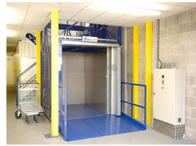
Product Load Elevator
